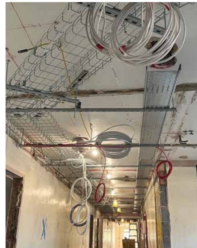
Caption: The electrical cables
